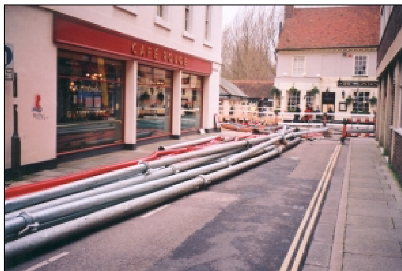
Figure 3 A pumping operation was successful in preventing major flooding of Chichester.
