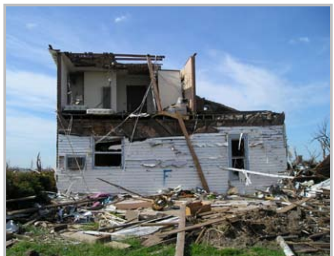
Damage to a residential structure from an F5 tornado that struck Greenburg, Kansas in May 2007
