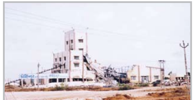
Salt factory damage caused during the 2001 Gujarat earthquake
